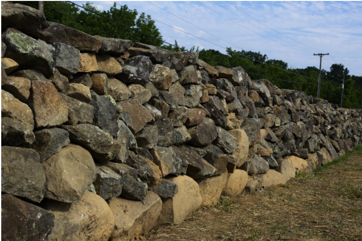
As part of the park's effort to return the battlefield to its 1863 character, dry-laid stone walls are currently being restacked in accordance with National Park Service guidelines. Photo courtesy Kevin Aughinbaugh.
