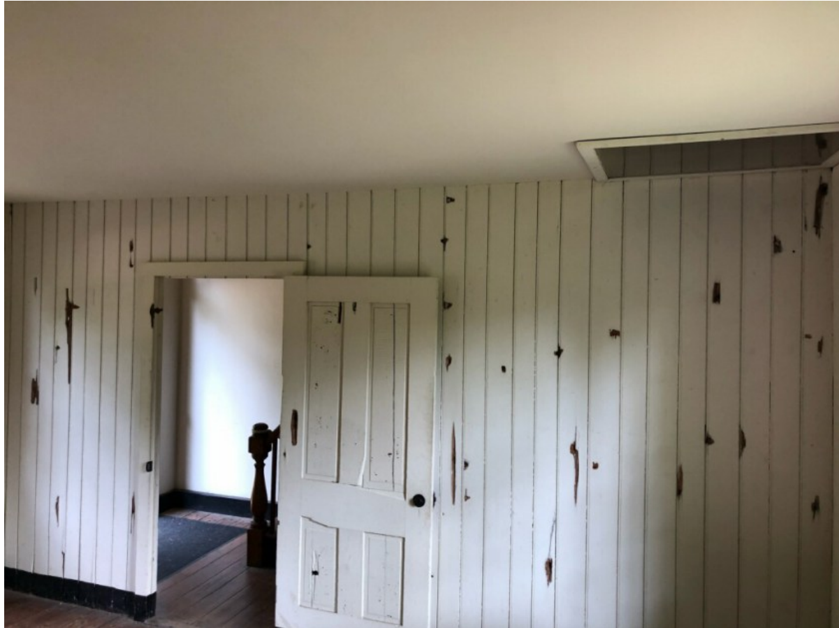
This picture of the parlor wall of the Innis House shows the bullet holes that still scar it. These were made by just some of the thousands of bullets that flew through the air each minute during the Battle of Fredericksburg. Photo courtesy Zach Wesley.
