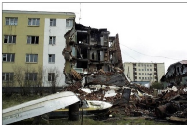
Damaged building infrastructure due to permafrost thawing in Siberia
