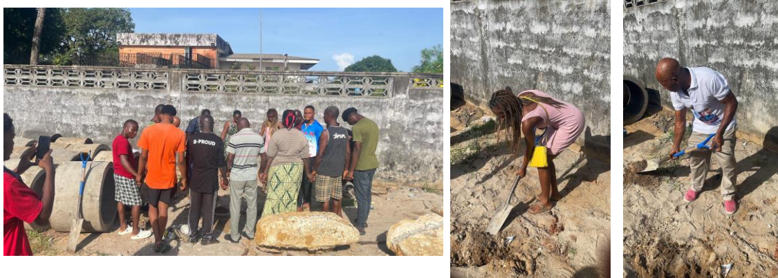
Figure 5: Pictures of the traditional groundbreaking ceremony with leaders of Yeakpee town community (the grey circular blocks on the far left are culverts purchased to begin the work).
